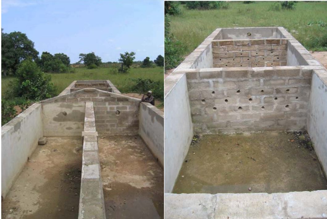
Figure 81 UNICEF HRF in construction at the Chirifoyili Dam, Northern Region Ghana Photo Credit: Jen Christian-Murtie, 2007
