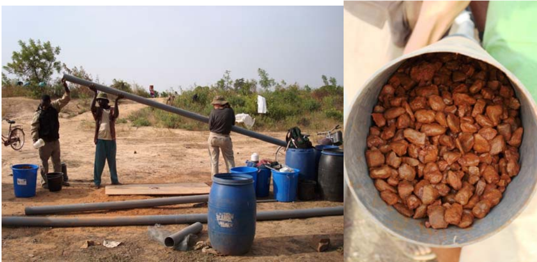
Figure 54 Filling pilot HRF tube with media (left), fully packed D tube with media (right)
